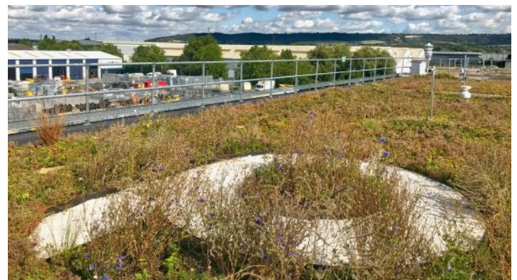
Blue green roof, New Hythe, Kent Photo: Polypipe
